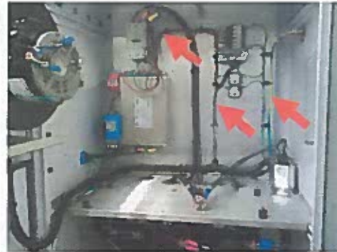
Controlled Wire Routing
